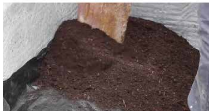
With the land drain protected, backfill with soil or other substrate as required.
