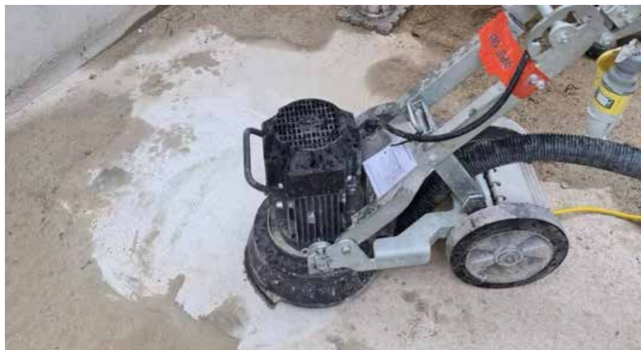
To prepare the horizontal areas, a diamond grinder or powerful jetwasher should be used.
