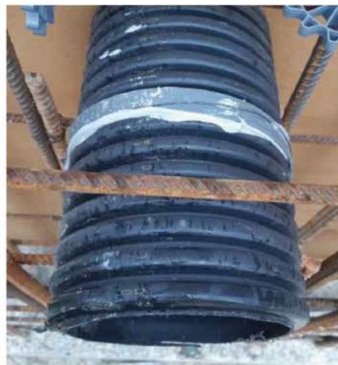
RIBBED PIPE Fill ribs with Hydrostop WSM. Apply Hydrostop WS10 to pipe using tying wire to secure. Overlap waterbar by 75mm side by side. Position to maintain a minimum of 75mm concrete cover.
