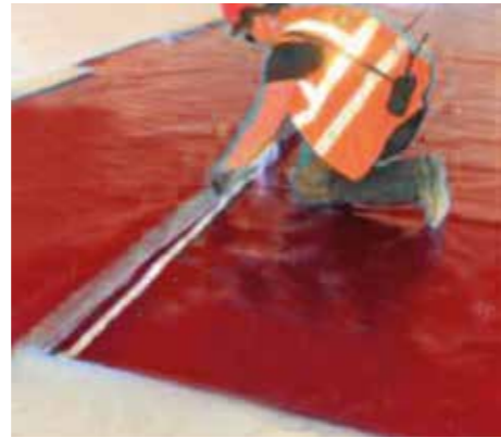
Laps sealed using HCR Butyl Tape between lap and HCR Foil Girth Tape overlap.
