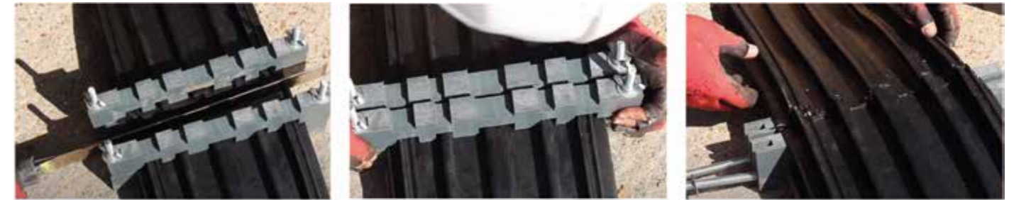
Position the hot knife between the ends of the Hydrobar and slide the second Hydrobar into the hot knife.
