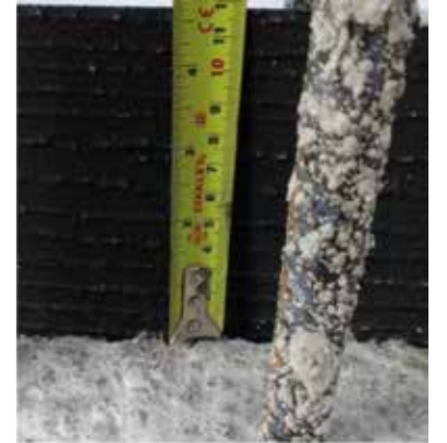
Ensure waterbar is installed with 30mm embedment into first pour, leaving 120mm protruding for wall pour.
