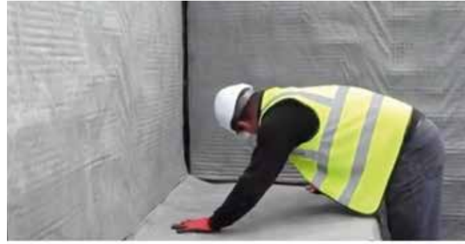
Only apply to horizontal surfaces where it remains continuous and directly joined to vertical sections, ensuring effective water management without unnecessary exposure.
