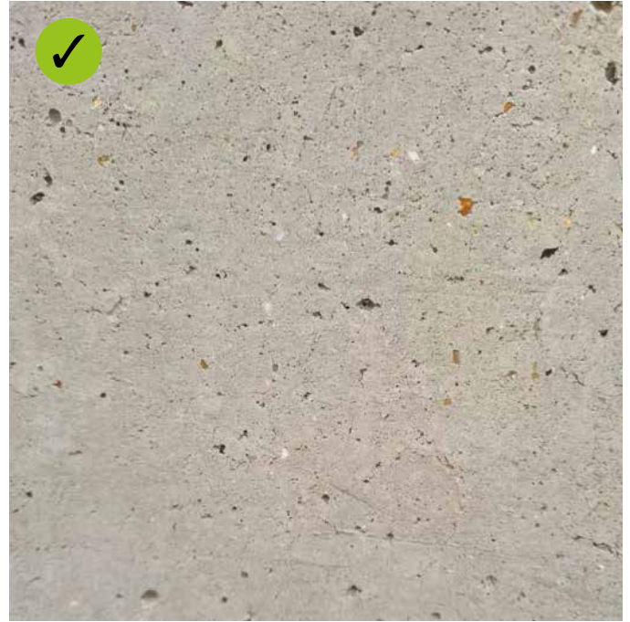
Example of suitably prepared wall. Note that the surface is rough and aggregate exposed.
