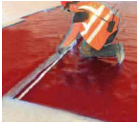
Laps sealed using HCR Butyl Tape between lap and HCR Foil Girth Tape overlap.
