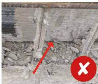
There must be no gap beneath the Cemflex VB after the first concrete pour.
